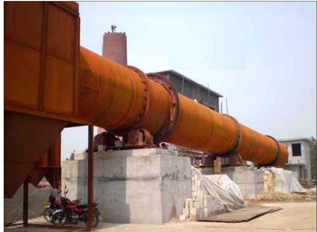
Rotary calcining kiln
